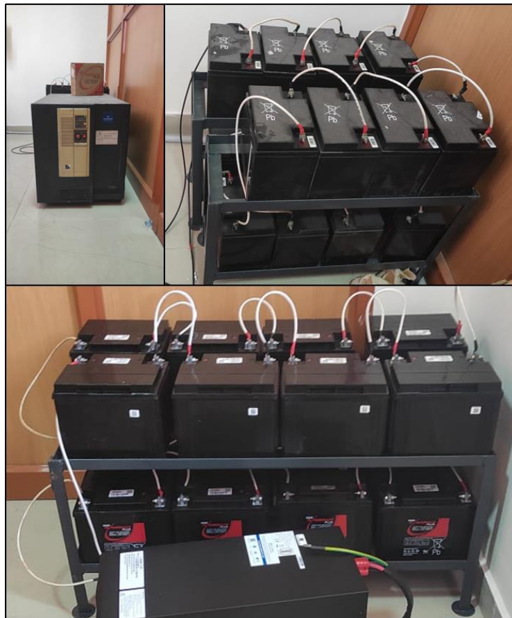
UPS System Facility at Sri Saradha College for Women
