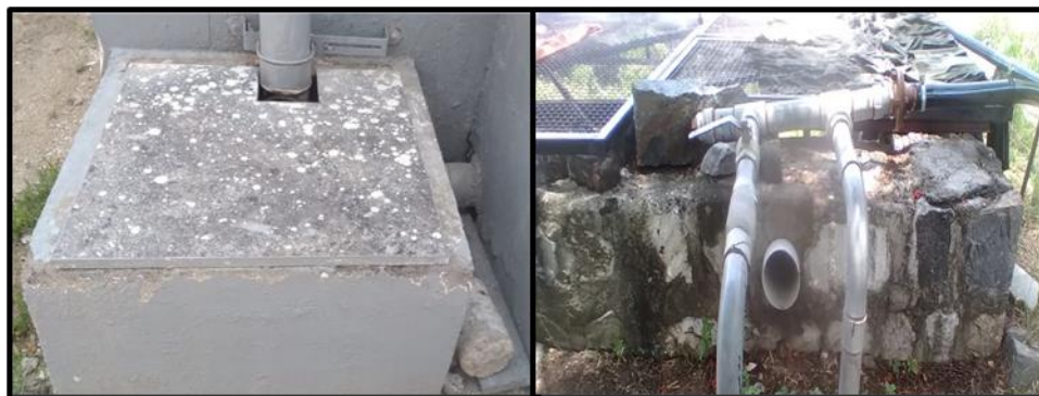
Rainwater harvesting system Found in the Campus
